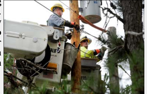
Atlantic City Electric line workers install a new utility pole, transformer, and tree-resistant aerial cable to improve service reliability for Cumberland County customers.
