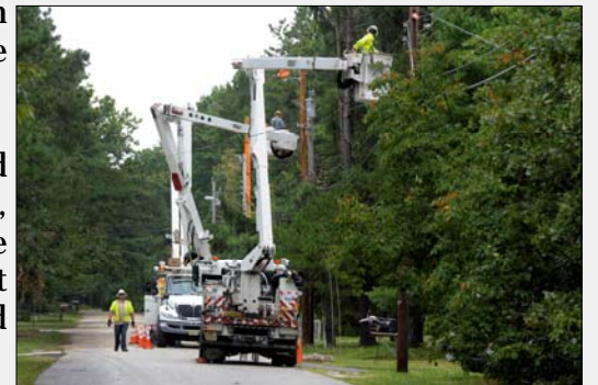
Atlantic City Electric crews complete reliability enhancement work in a Bridgeton neighborhood to modernize and strengthen the local energy grid for area residents.
